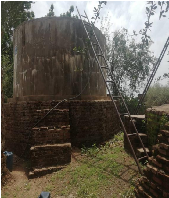
Figure 33: Water tank at one of the visited sites
