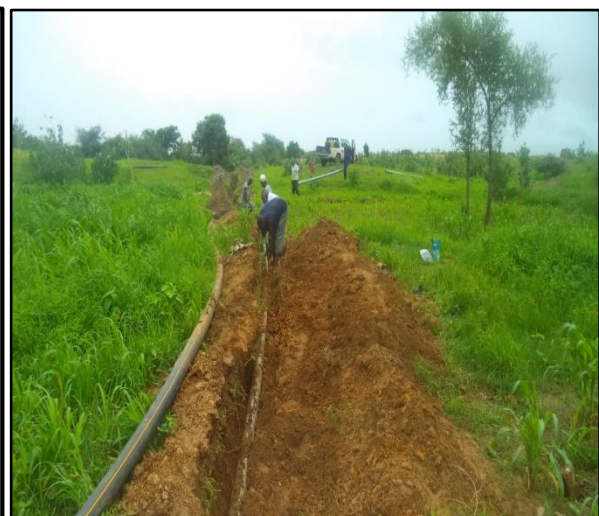
Figure 5: Water committee repairing water pumping line in Hassa Hissa camp, sector 2 (CDS)
