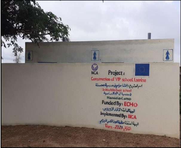
Figure 22: Lockable VIP latrine for school girls at one of the schools, for their privacy
