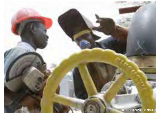
Worker welding firefighting equipment at a petrol depot in Dar Es Salaam.
