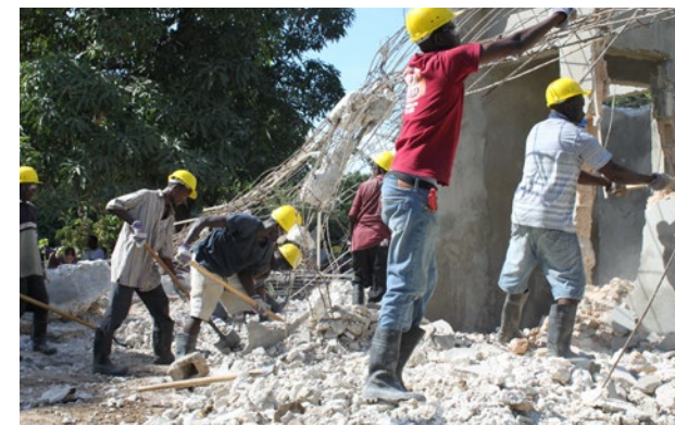
Removal of debris from the streets of Port-au-Prince and Léogâne in November 2011, nearly two years after the 2010 earthquake. PHOTO: UNDP/Flickr
