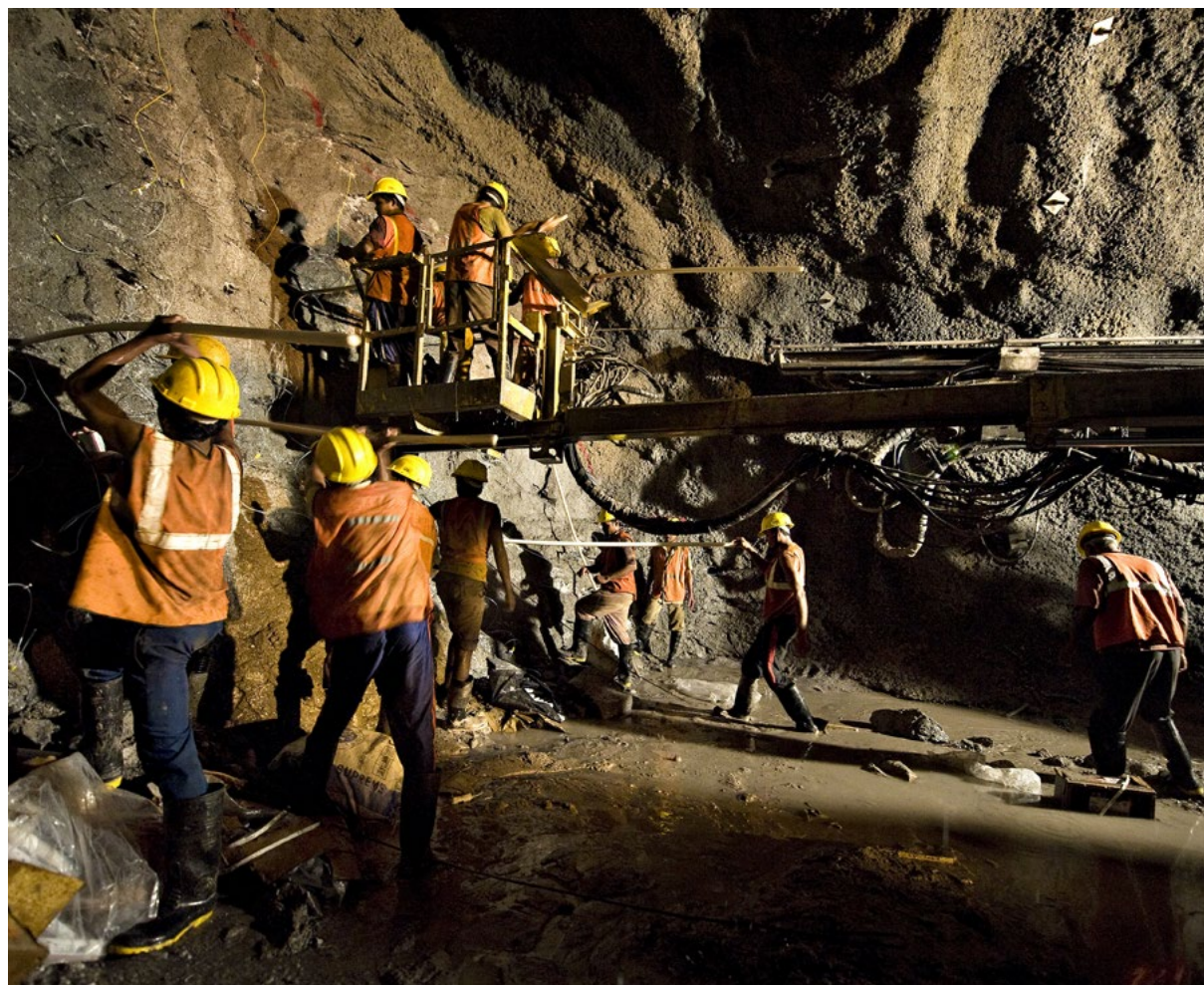
The team who drill holes and load explosives are preparing the next blast in Punatshangchhu in Bhutan. PHOTO: Ken Opprann
