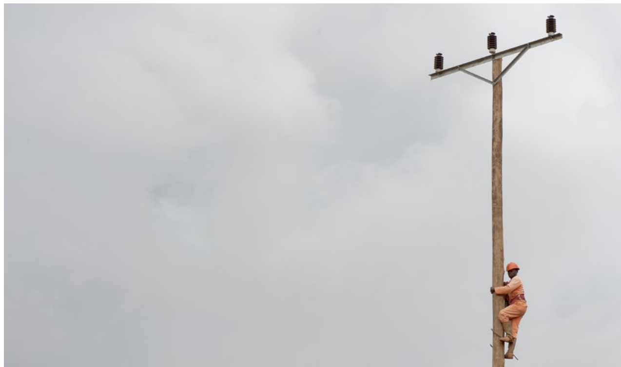
Assembly of power poles outside of Lichinga in Mozambique. PHOTO: Ken Opprann
