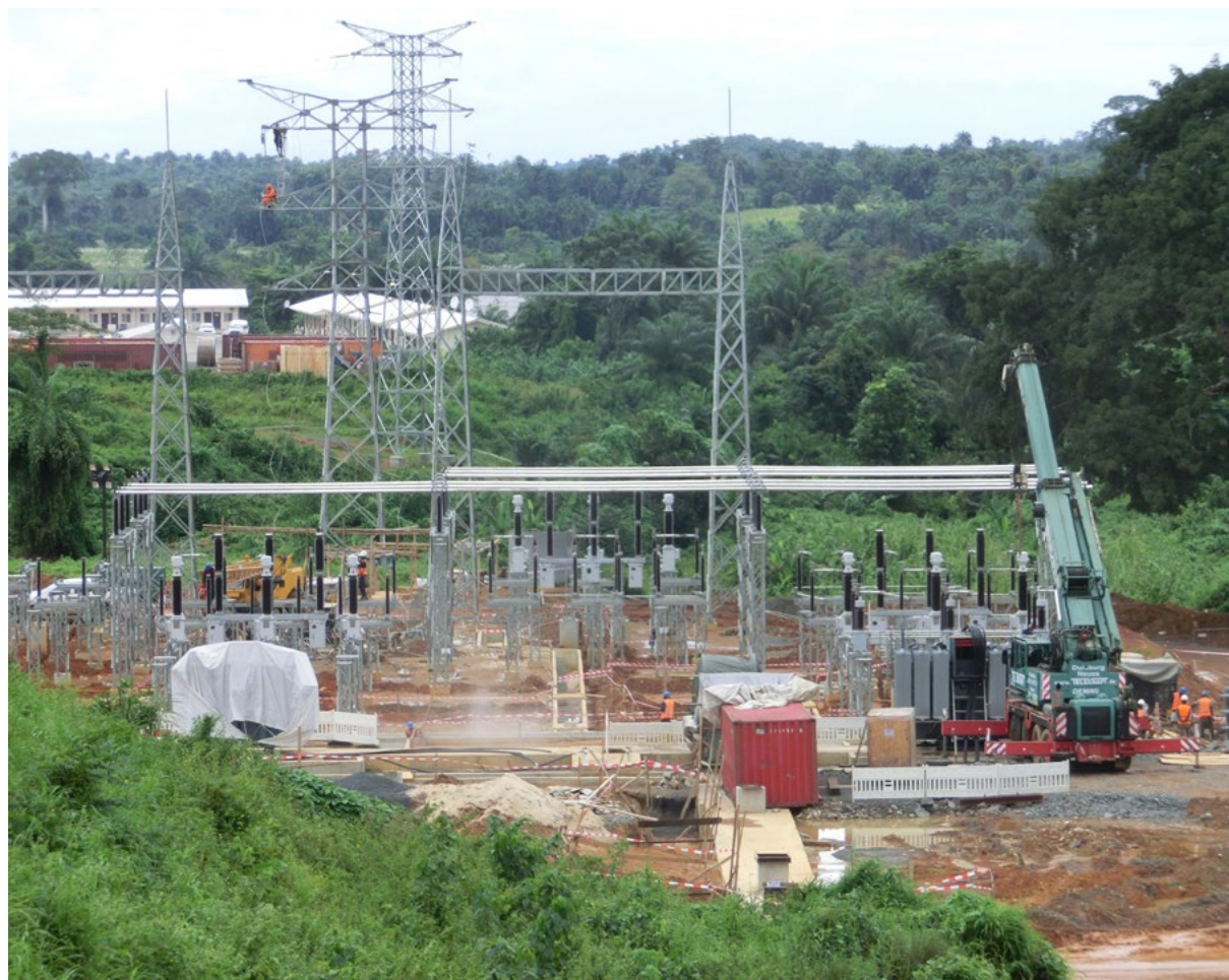
Transformer and switching systems under construction in Monrovia, Liberia. The plant distributes power from Mt. Coffee power plant out on two 66kV power lines to Monrovia. PHOTO: Knut Gakkestad
