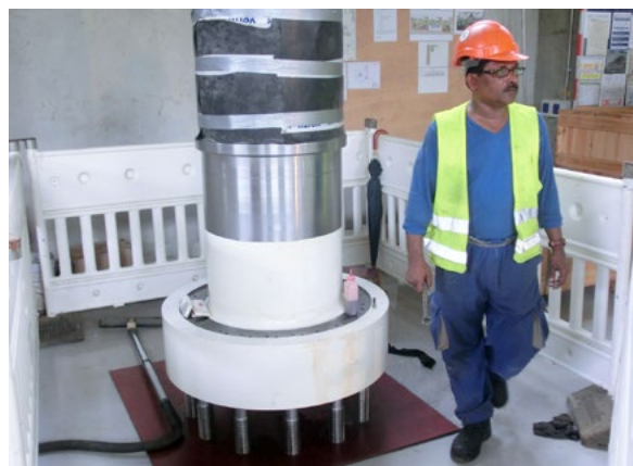
Preparation of turbine shaft for mounting on Mt. Coffee power plant. PHOTO: Knut Gakkestad
