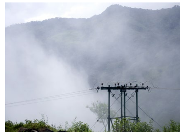
Power line in the mountains by the Tala dam in Bhutan. PHOTO: Ken Opprann
