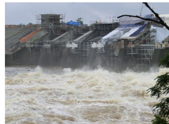
Rehabilitation of the 10 flood gates from 1964 at the intake dam to Mt. Coffee power plant. PHOTO: Knut Gakkestad
