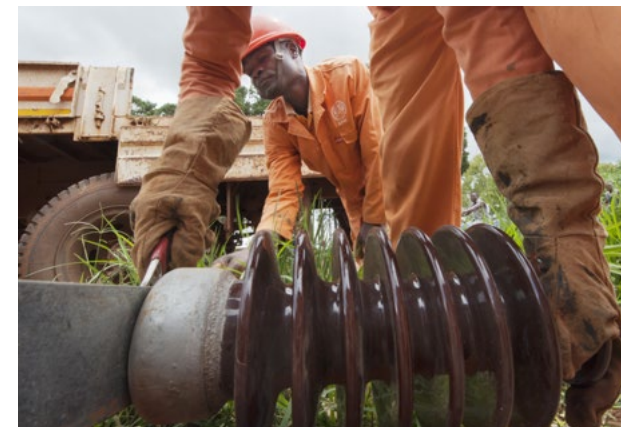
Assembly of power poles outside Lichinga in Mozambique. Norway has cooperated with Mozambique within the energy sector for the past 40 years. PHOTO: Ken Opprann
