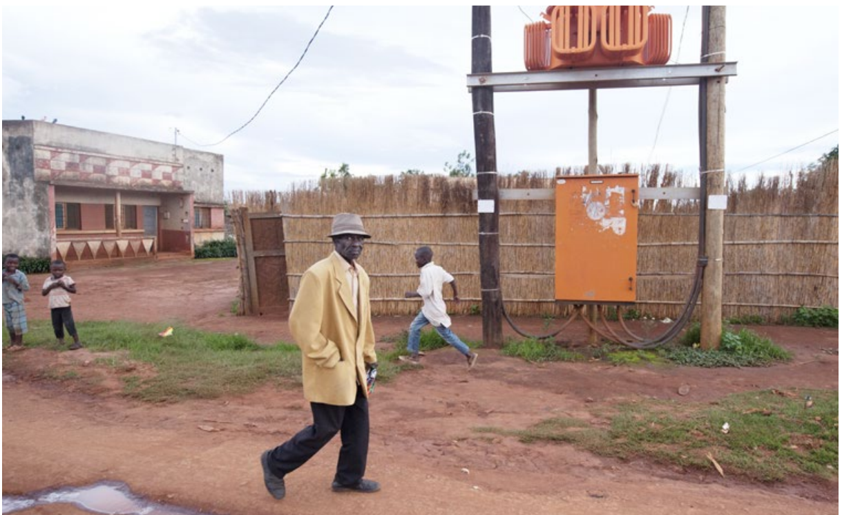
EDM's characteristic orange distribution transformer now symbolises access to electricity and development. PHOTO: KEN OPPRANN
