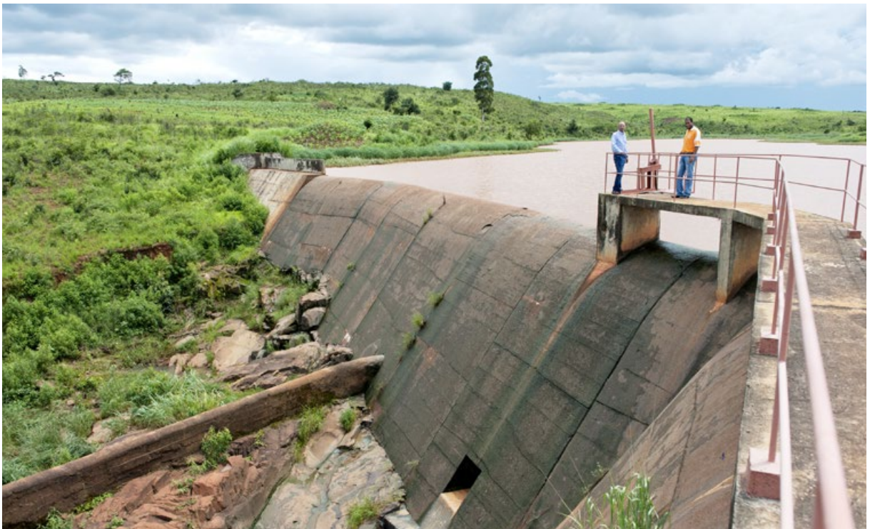
2017: Lichinga small power plant. The finished dam, still in operation. PHOTO: KEN OPPRANN
