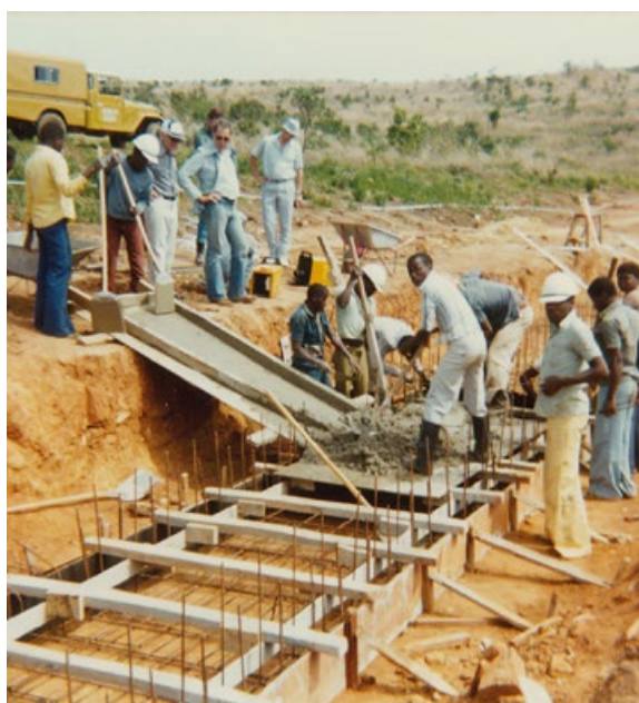
Engineers from EDM and Norwegian experts carrying out an inspection in connection with the construction of the small power plant in Lichinga in Northern Mozambique early in the 80s. PHOTO: NORAD'S ARCHIVES
