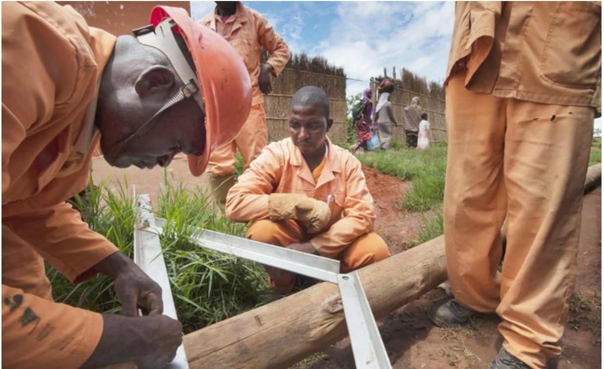
EDM technicians constructing poles during installation of a power line in Northern Mozambique. PHOTO: KEN OPPRANN
