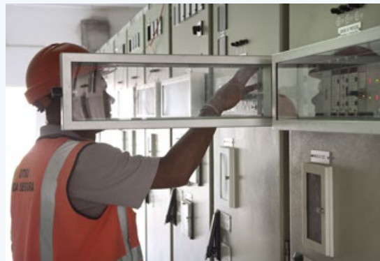
The connection station CTM supplies electricity to Mozambique's two largest cities. The images show parts of the old station that is undergoing an upgrade. PHOTO: KEN OPPRANN
