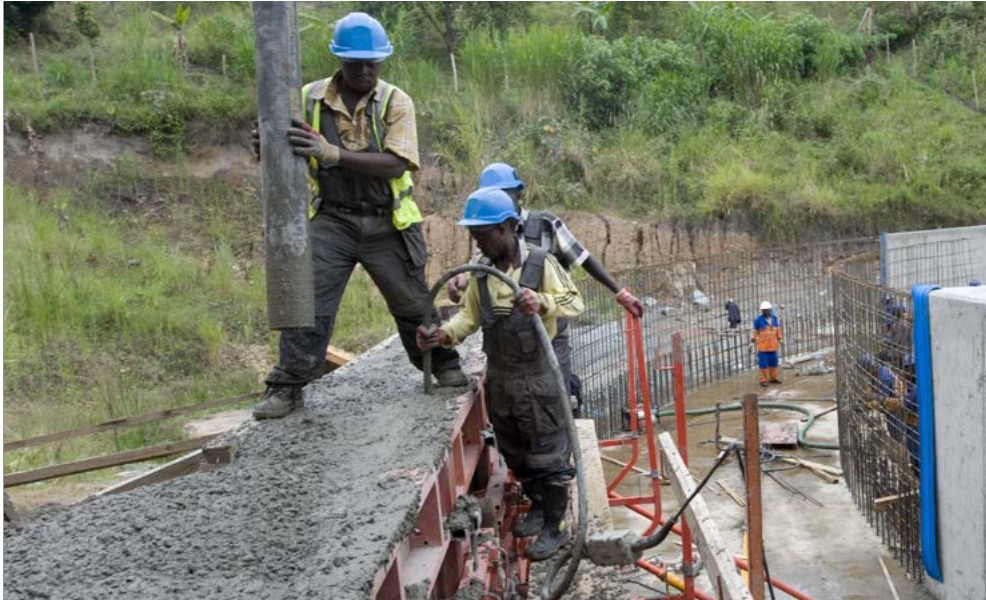
Construction of Bugoye created many local jobs. Here construction workers fill the walls of the canal. PHOTO: KEN OPPRANN
