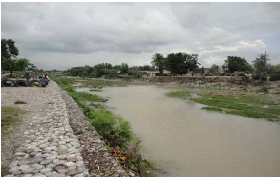
Figure 4 Photo: River bank protection at the lower 'Grande Ravine du Sud' near Les Cayes
