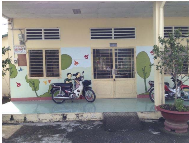
Good example of an additional ramp leading to classrooms. Unfortunately the tiles in use are very slippery when wet.
