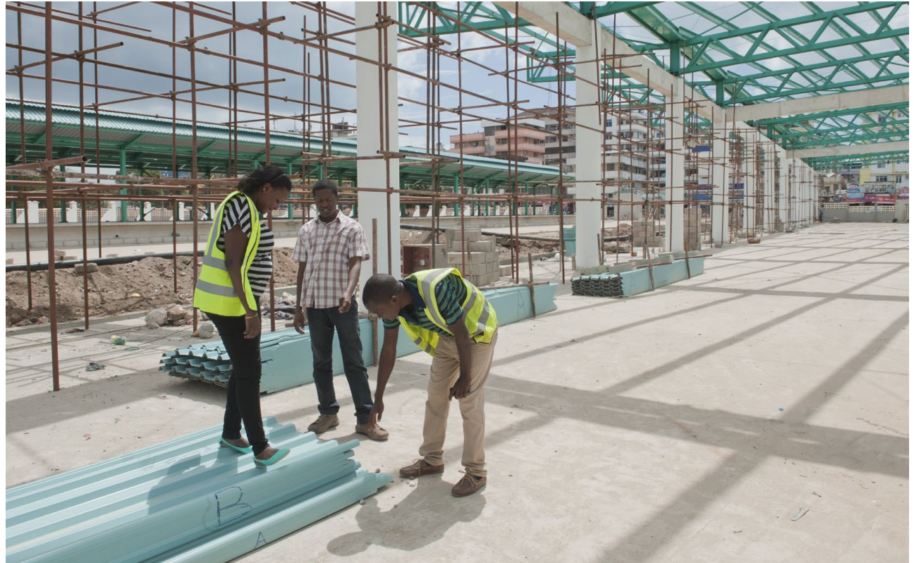
Engineer Angela Genes with colleagues inspecting the construction of the new bus station in Kariakoo, 2015. FOTO: PHOTO: KEN OPPRANN
