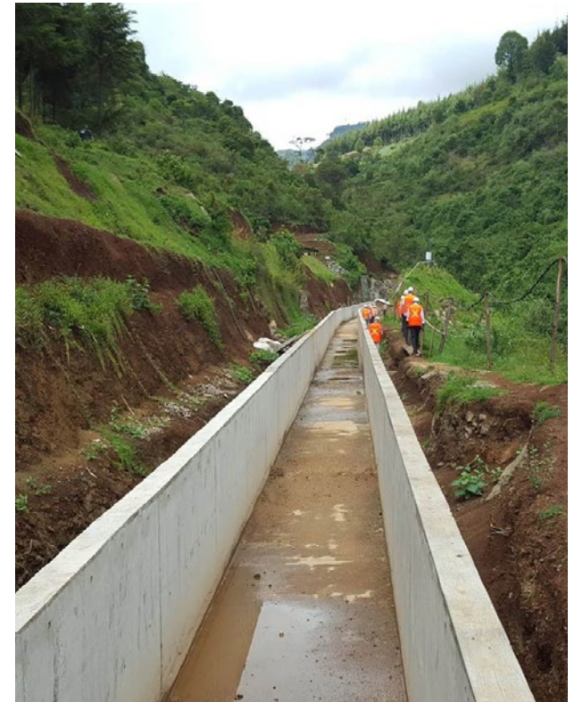
Construction on the 6.3 MW Siti I HPP which is being realized as a consequence of the GET FiT Program PHOTO: FRONTIER INVESTMENT MANAGEMENT
