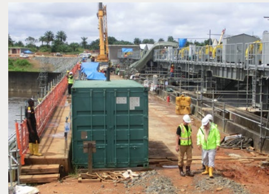
Mt. Coffee HPP spillway dam, refurbishment of flood gates. PHOTO: KNUIT GAKKESTAD
