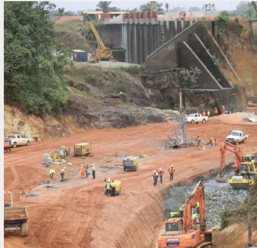
Construction is underway on the 88 MW Mt. Coffee hydro power plant. PHOTO: KNUT GAKKESTAD
