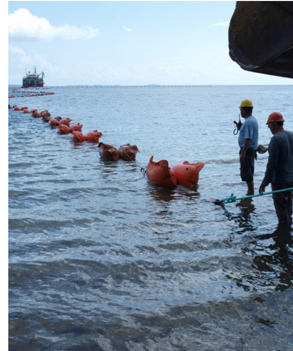
Work on the 73-kilometre subsea cable connecting the island of Pemba on Zanzibar to the Tanzanian main grid. PHOTO: MULTICONSULT
