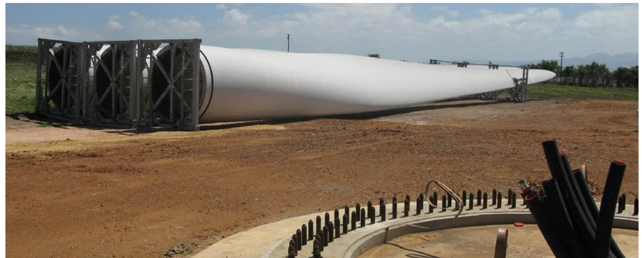
Windpower turbine foundation at Kouga Wind, South Africa. Rotor blades ready for installation in the background. PHOTO: GEEREF
