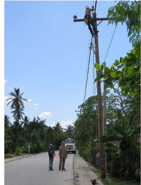
The mini-grid in Coteaux PHOTO: UNEP
