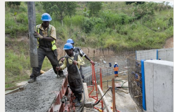
Construction of Bugoye created many local jobs. Here construction workers fill the walls of the canal with concrete. PHOTO: KEN OPPRANN
