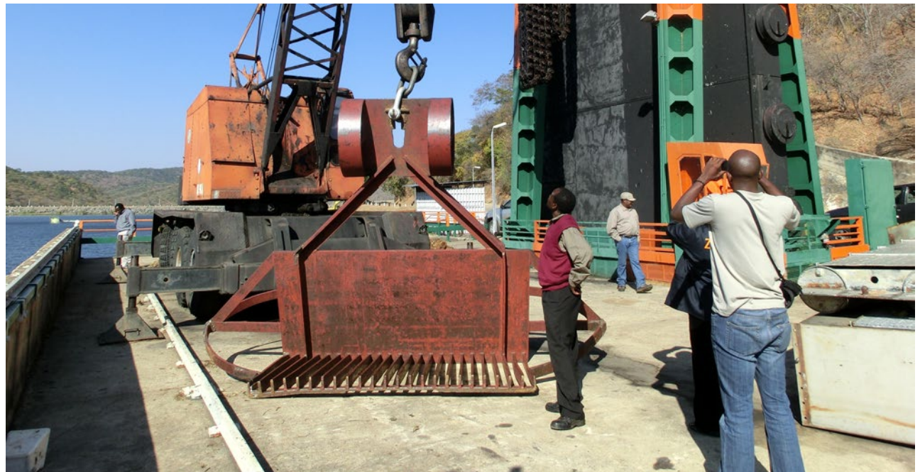
Kafue training centre. Facilities for practical training. Maintenance of intake gates. PHOTO: KNUIT GAKKESTAD
