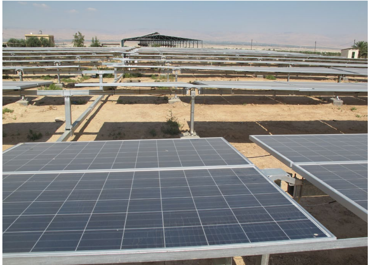
Solar power plant in Jericho, Palestine. PHOTO: HARALD BIRKELAND
