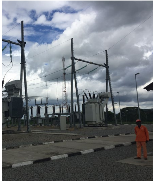
Norwegian funded trafo station in Cabo Delgado region PHOTO: ENDRE OTTOSEN
