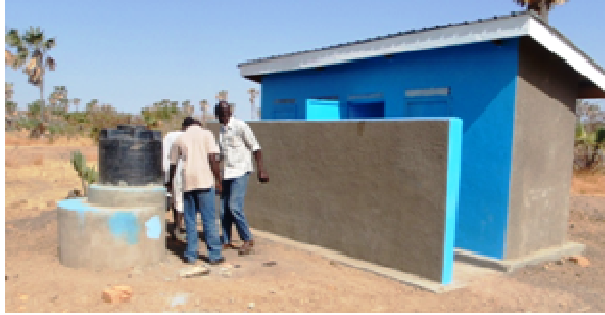
Plate 6 – A Completed institutional latrine at Nyokithian primary school with hand wash facility
