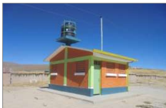
Image N° 3: Protective Metal Framework of Water Tank – Iracachi Sanitary Unit
