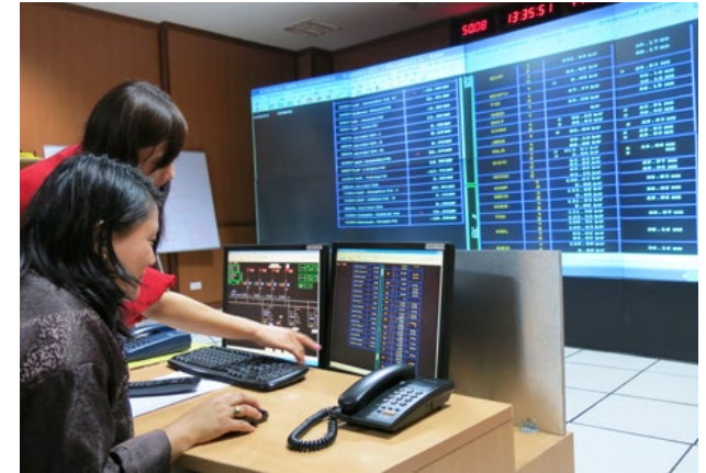
The control center of Bhutan Power Corporation. PHOTO: ENDRE OTTOSSEN
