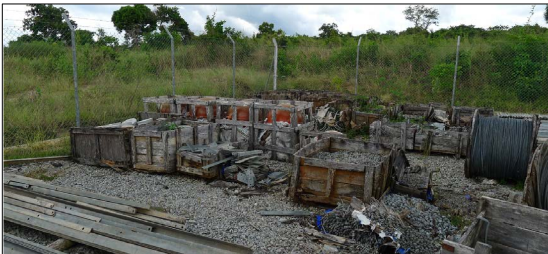
Picture 2. Storage of surplus parts from the installation works in Macomia substation.
