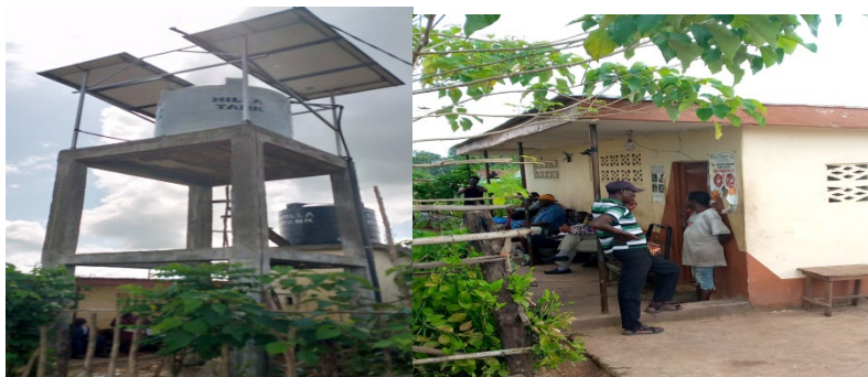
Figure 4.4a: Installation of solar borehole as an unintended positive outcome at Tiama toilet project site by council
