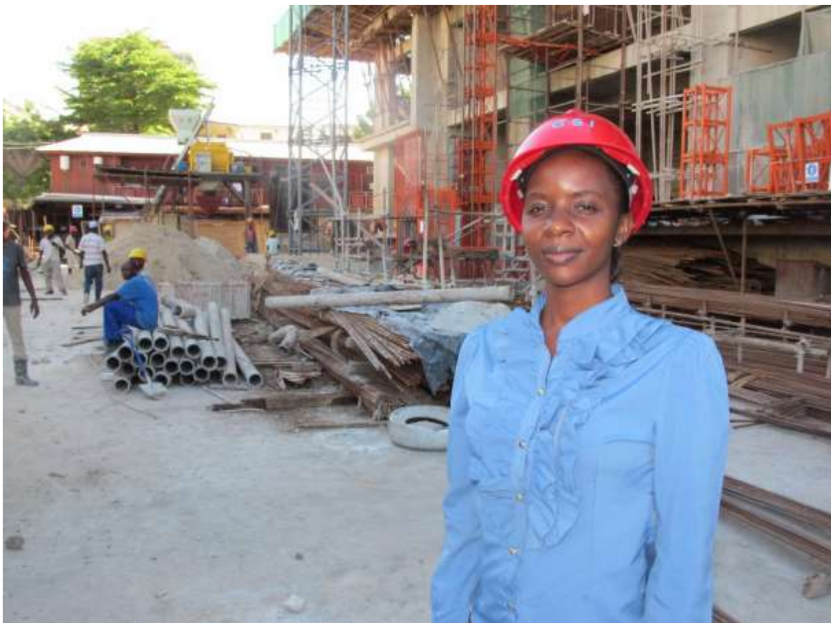
SEAP trainee Martha Daniel supervising workers at a construction site in Dar es Salaam.
