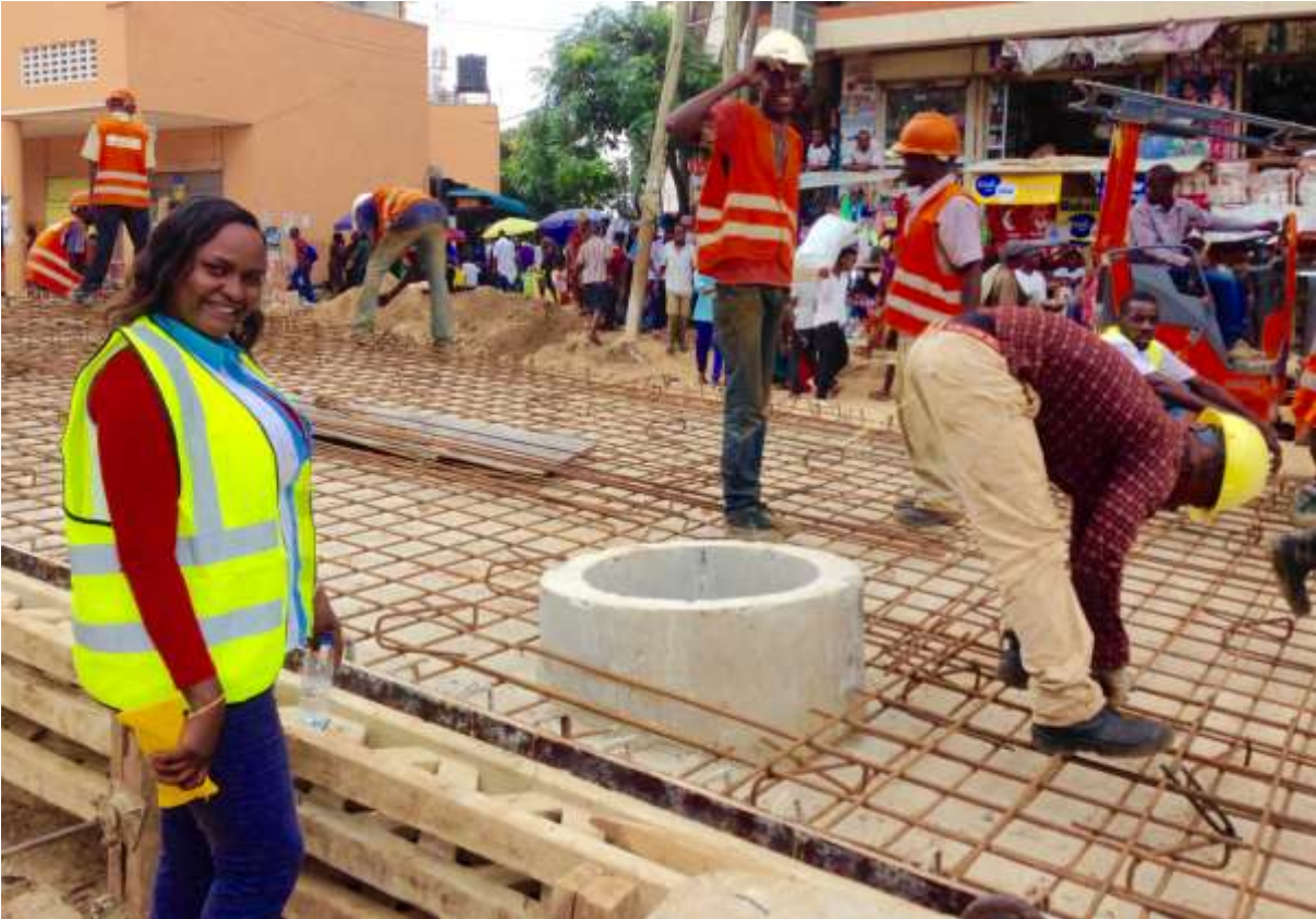
SEAP trainee Angela Genes supervising workers at construction site in Dar es Salaam.
