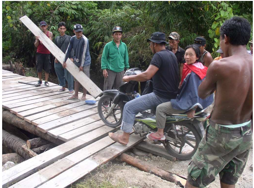
Evaluator on ojek to Sirilaggai. Villagers repairing bridge destroyed by flood (Pix: Andreas)
