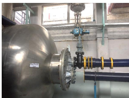
Figure 14 new turbine under installation at the Turbine Testing Lab at Kathmandu University
