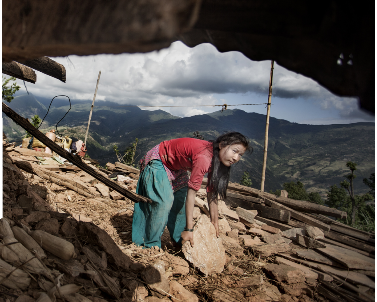
A woman rebuilding her house in a mountain village 2600 metres above sea level north-east of Kathmandu after the earthquake in 2015. PHOTO: ØYVIND NORDAHL NESS / VG
