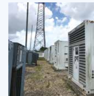
The diesel generators at Mtoni, Unguja. Photo: Multiconsult (2019)
