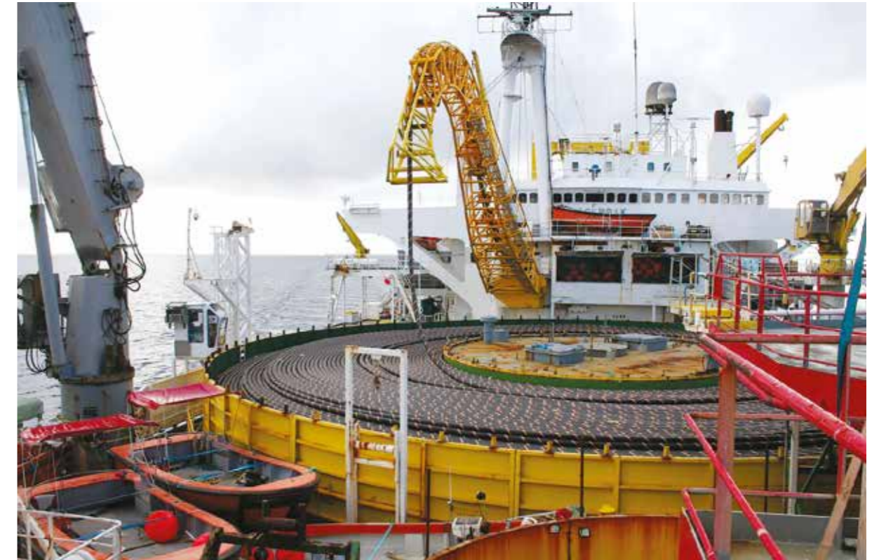
The 77 km long sub-sea cable to Pemba on the boat, ready to be unwound into the sea. Photo: John Alvsvåg (2009)
