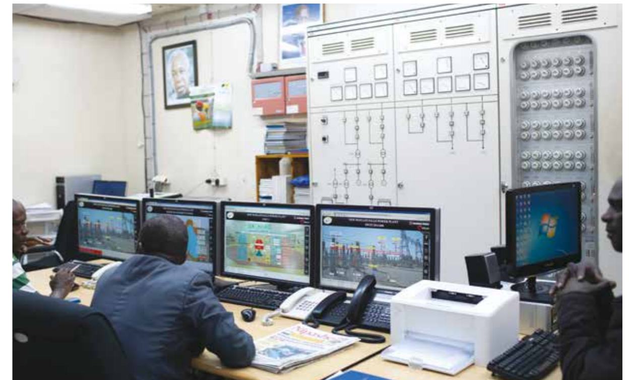
Following the repair and capacity building programme supported by Norway, outages were reduced from 170 hours to only 8 hours during a month. Photo: Espen Røst (2019)
