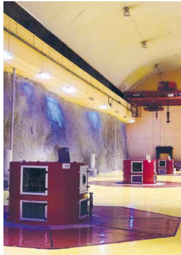
Kihansi Power House. Photo: Espen Røst (2019)
