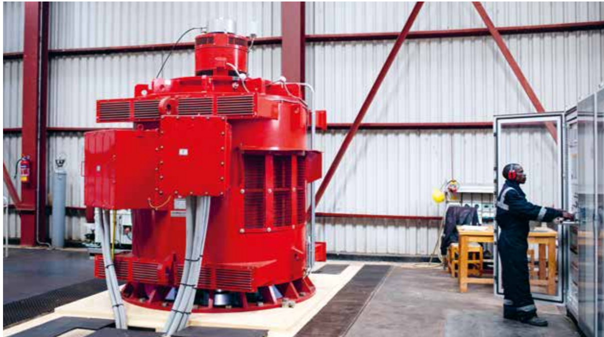
Joffrey Kisonga has worked as an operator for the last seven years at the privately owned Mwenga hydropower plant (4 MW) in the Iringa region. He operates and maintains the plant, ensuring smooth daily operations. Photo: Espen Røst (2019)
