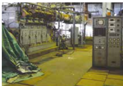
Old IDO generators. Photo: Solveig Middtun Bæra (2019)
