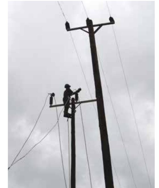
ZECO employee Omar Ali climbing the power poles at Mbagadu in Pemba: The distribution lines are being upgraded from 11kV to 33kV, as part of the Capacity Building on Maintenance Project supported by Norway. Photo: Solveig Midttun Bæra (2019)
